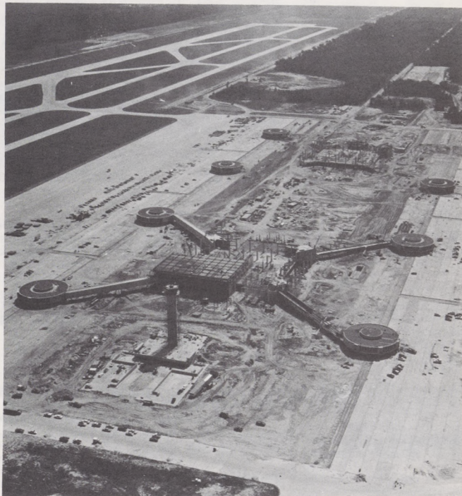
The new type FAA tower stands tall at Houston Intercontinental Airport where the runways are finished and buildings are taking shape.
