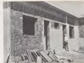
Above, this rather slapdash looking building at Biga, Turkey, houses highly sensitive VOR equipment.
