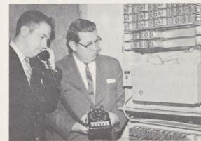
If all the specialists are busy when a pilot calls the FSS, this new DCA equipment notifies the pilot with a recorded message that his call has been received.
