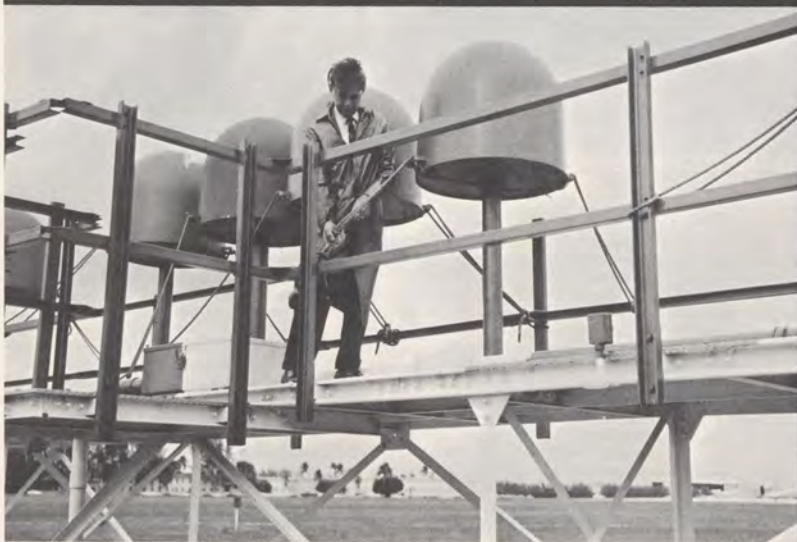
AFS chief Jule McDowell ties down ILS localizer antenna at end of a Miami runway.
