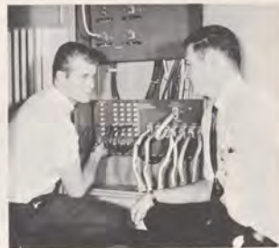
Technicians check radar patch panel.
