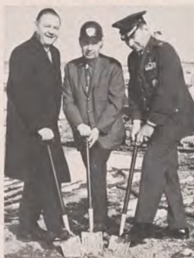
Ground was broken for a combined air traffic control tower and radar approach control facility at Elmendorf AFB, Alaska, by, from left, Alaskan Regional Director George M. Gary, Swalling Construction Company president Albert C. Swalling and Colonel Olin E. Gilbert, Alaskan Air Command. The cost is over $1.4 million.
