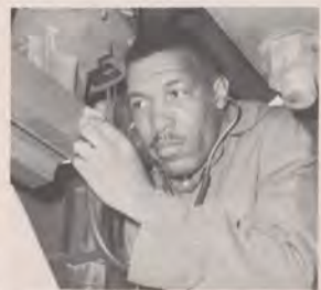
Technician Warner Turner uses a stethoscope to check antenna drive gear assembly at Washington National.
