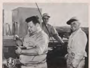
CE's Edward L. Johnston, August J. Schmidt and Thomas C. O'Conner install rooftop beacon to guide pilots.
