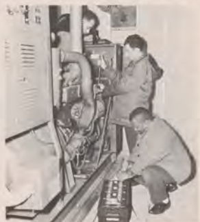
Technicians Seymour Chenkin, Sebastian Virga and David Powell of the LaGuardia Airway Facilities Sector install a battery on a 75 kva generator for an ASR-4.
