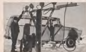
Frank S. Fields and Toivo Olsen install Short Approach Lighting System at Bethel, Alaska, to aid pilots when snow and overcast obscure the horizon.
