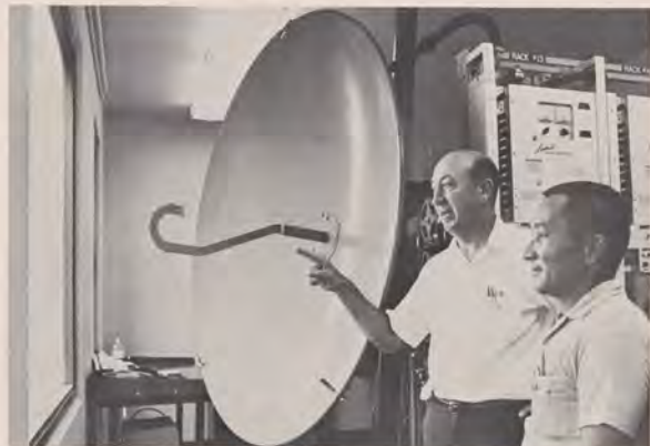
Pointing to a plastic "picture window" in Kahului Airport's combined station-tower through which Pacific Region's only indoor micro-wave dish antenna beams its signal to an air-ground station on 10,023-foot Mt. Haleakala, is Charles Miesel, Airway Facilities chief, Maui, with EMT Suetoshi Tamanaha.
