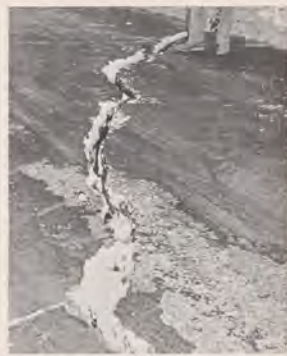
Taxiways took a beating from tembor that hit Aleutian chain last February. Damage to facilities was slight.
