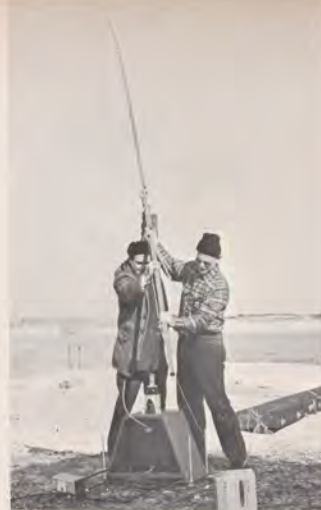
A 35 foot antenna was swung into place by Lloyd Boggs and Art Moskowitz as the Eastern Region Accident Support Team used an FAA transceiver to link the FAA Region and the accident site.
