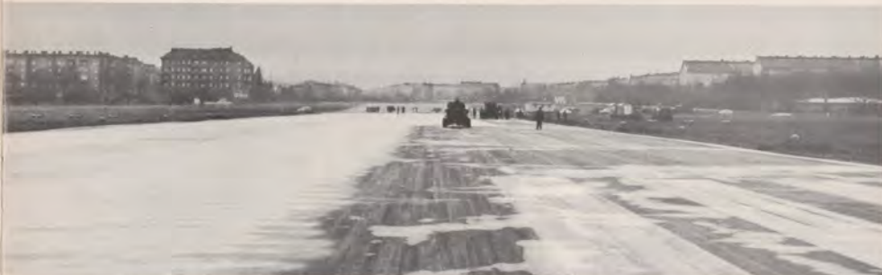
This view shows the approach end of runway 27L and the buildings flanking each side. Men and equipment are engaged in resurfacing the runway.
