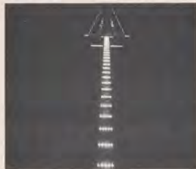
The Federal Aviation Agency has cut minimum visibility at Metropolitan Oakland International Airport to 2,000 feet because of greater safety of the new lighting system.
