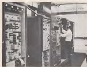
Southern Region SMS electronics technician, D. E. Sullivan at work inside the Crestview, Fla., VORTAC.
