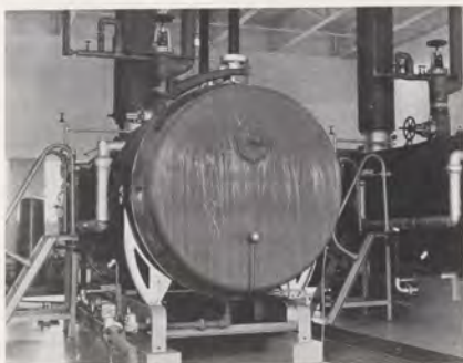
Huge boilers heat water to sterilization point (approximately 180 degrees F).
