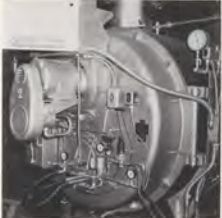
Fire control end of huge boiler.
