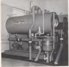
Water is pre-heated before being boiled.
