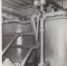
Rain water is pumped through these filters.
