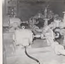
These pumps force water to ready tanks.
