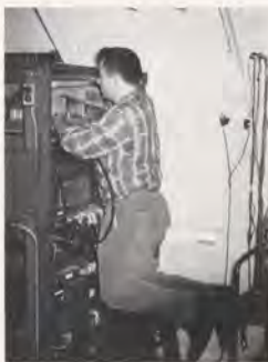
Technician working on rack holding transmitting and receiving equipment for 272.2 megacycles, a task requiring the highest skill.
