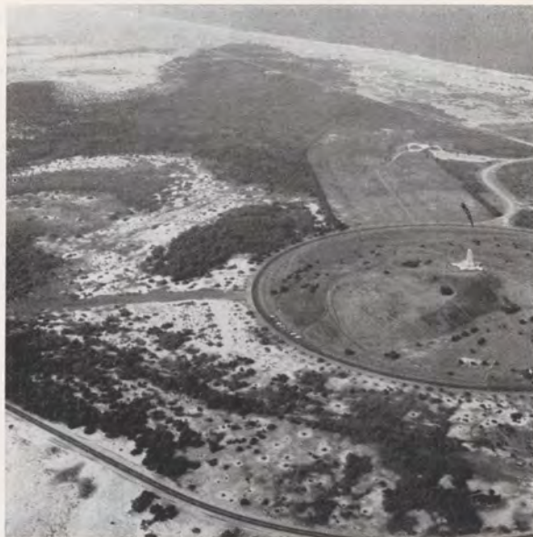
This is the site of the new 3,000-foot-long, 50-foot-wide landing strip under construction at Kitty Hawk, N. C., where man's first powered flight was made. On December 17, 1963, the 60th Anniversary of Orville and Wilbur Wright's flights, impressive ceremonies will be held saluting this memorable achievement.
