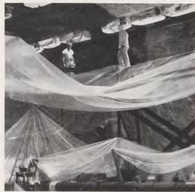
Unusual effect is created during painting of ceiling in control room of Oakland ARTCC at Fremont. Plastic "draperies" protected sensitive equipment from paint, providing an effect akin to that one would expect in a science-fiction movie.
