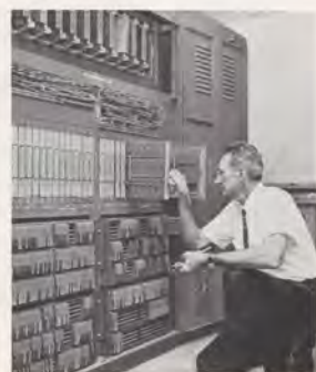
Gene Gaither checks the "innards" of a control panel.
