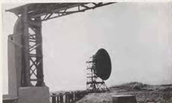
The troposcatter system at Middleton Island is the first of its type to be operated by FAA.
