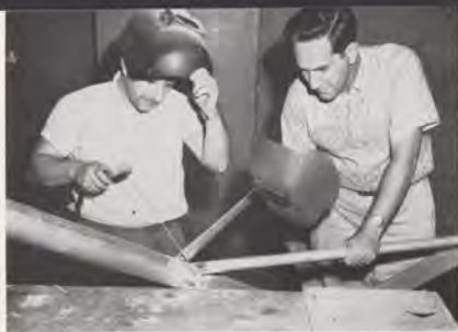
Repair of a base structure for a remote radar site eliminates time-consuming commercial repair contracting. Michael S. Cirillo, Machine Shop Leader (right) is assisted in a repair spot weld by Tony Savarese on an antenna light mounting.
