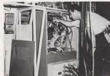
Nav aids, radar, communications and power plant systems connect like arteries into the IFR room at New York International Airport. Electronic specialist Leonard Gettsfeld, SMS-33, reflects the "inward" of one of the components vital to the functioning of the radar track.
