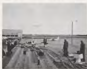
After the treacherous winds subsided, leaving a wake of destruction, workmen from SMS-92 and airport men wasted no time in putting up a brand new roof.
