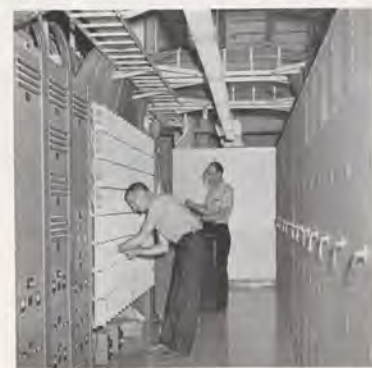
Cecil Howard (l) and Harry Johnson, Electronics Installation Technicians, work at frame in the communications equipment room.
