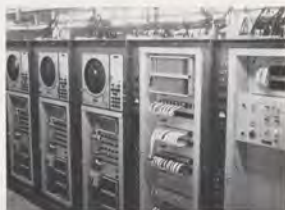
This photo shows part of the electronic equipment required to provide the controller with the information needed to control traffic. The equipment processes the beacon and radar information and converts it into a television type video presentation which can be displayed on receivers much like a home TV set.
