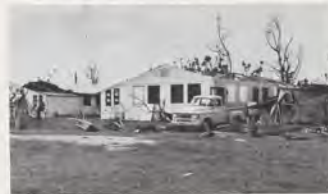
Aftermath of Karen—ruin. The demolished home of Manuel Marin, Supervisory Electronics Installation Technician.
