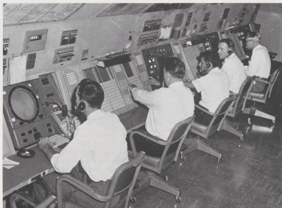
Installation of a 301 interphone system was completed in San Antonio Tower's IFR room. The approach control facility serves San Antonio International Airport, Kelly and Randolph Air Force Bases, and Stinson Field.
