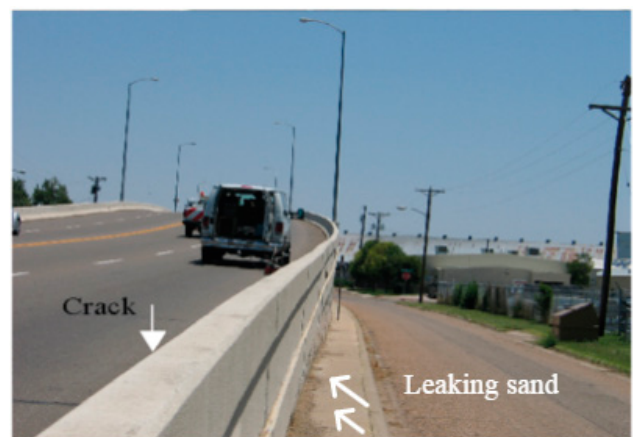
Figure 2.5 Leaking Sand From MSE Wall Due to Water Seepage (Adapted From D.-H. Chen et al., 2007).
