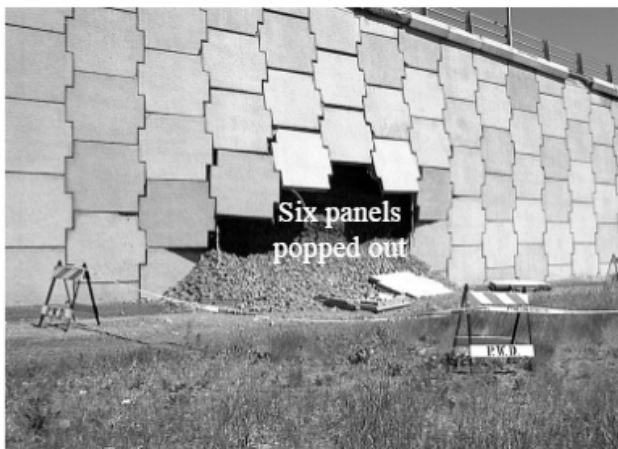
Figure 2.9 MSE Wall on Idaho State Highway 34. Panel Failure Due to Corrosion of Reinforcement (Adapted From Armour et al., 2004).
