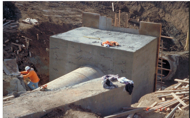
Figure 2.13 Leakage and Joint Rotation Adjacent to the MSE Wall at Highway 87 in Santa Clara Valley (Source: Hook et al., 2006).
