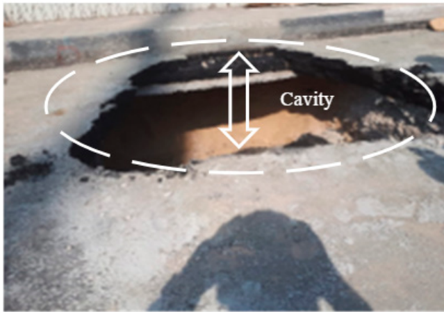
Figure 2.6 Pavement Collapse Due to Internal Erosion of MSE Backfill (Adapted From Kara & Tahoun, 2020).
