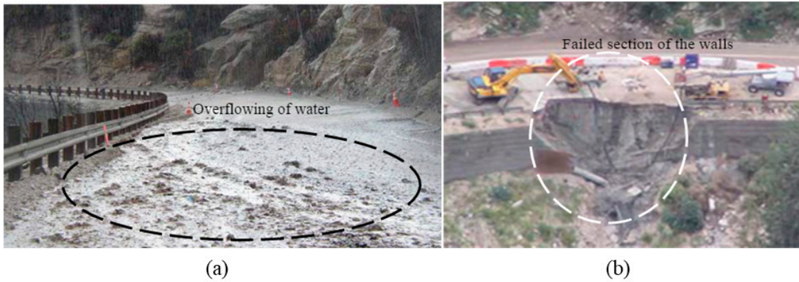
Figure 2.8 MSE Wall in Tucson, Arizona Displaying (a) Overflow of Water and Debris on the MSE Wall and (b) Failure Section of the MSE Wall (Adapted From Haramy et al., 2010).
