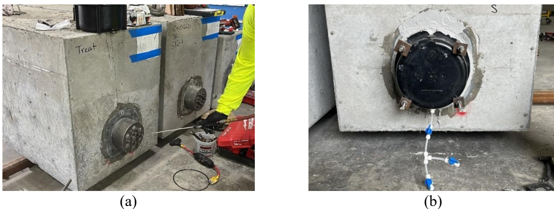
Figure 8.3. Preparing the PT live end of beam S12-P-T for impregnation of corrosion inhibitor: (a) Cleaning strands and anchorage end with compressed air; (b) Installation of customized end cap.
