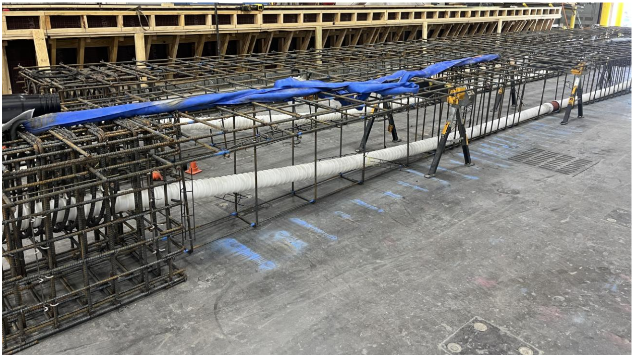
Figure 1.1. Assembly of reinforcement cages and ducts for the construction of a draped-tendon-profile post-tensioned girder.
