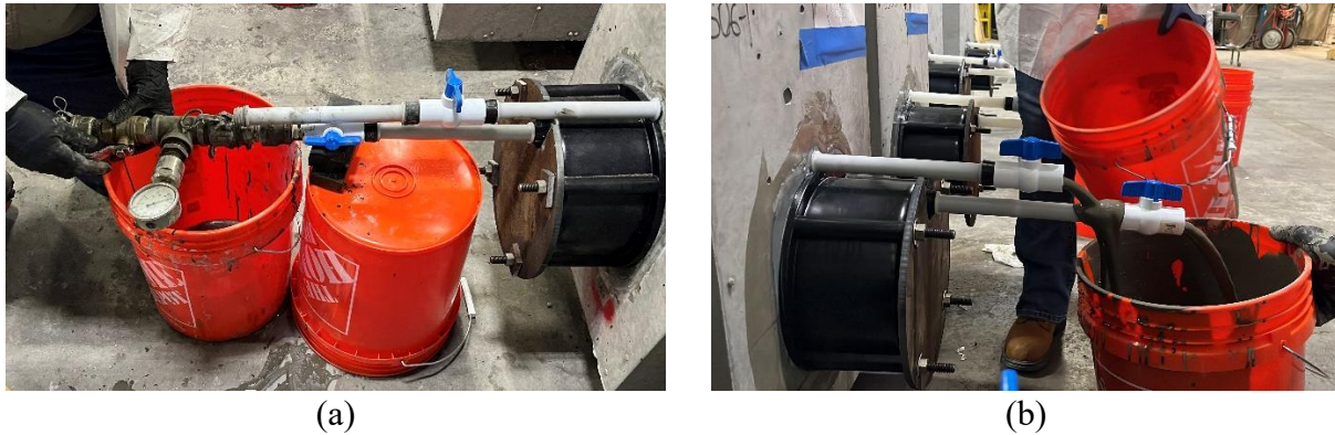
Figure 6.15. Grout injection of S06-M-TC beam in process: (a) Injection of grout at PT dead end; (b) Excess grout discharged at PT dead end grout ports.
