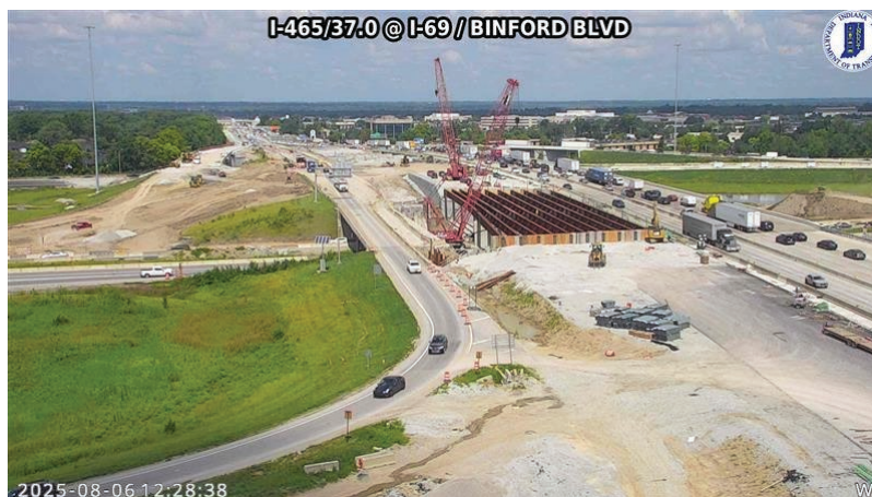
Figure 1. ITS Camera Image at the I-465 at Mile Marker 37, I-69, and Binford Boulevard Interchange showing the work zone configuration during the construction of a bridge.
