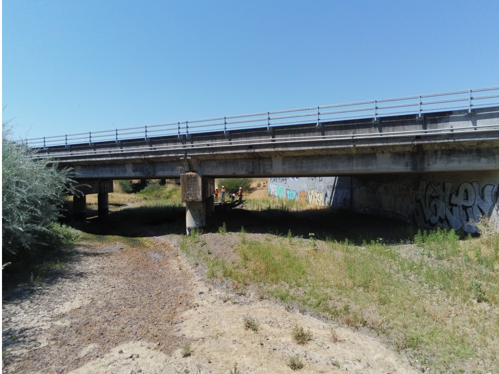
Figure 2.4: Overview of Bridge 1 (20 0019Y) (originally presented in the Task 1 and Task 4 reports).
