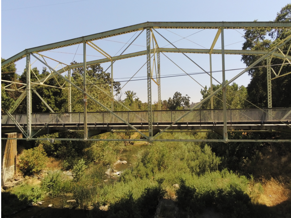
Figure 2.6: Overview of Bridge 2 (33 0046Y) (originally presented in the Task 1 and Task 4 reports).
