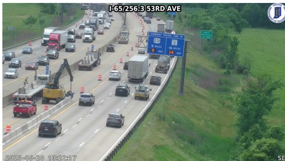
Figure 1. ITS Camera Images Along I-65 Near MM 256.3 on June 20, 2025 Showing the Installation of Temporary Concrete Barriers Next to Live Traffic.
