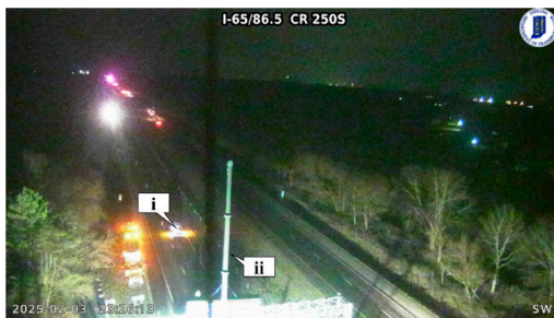
Figure 2.15 ITS Camera Image Along I-65 Near Mile Marker 86.5 Showing a DMS Sign Being Installed.
