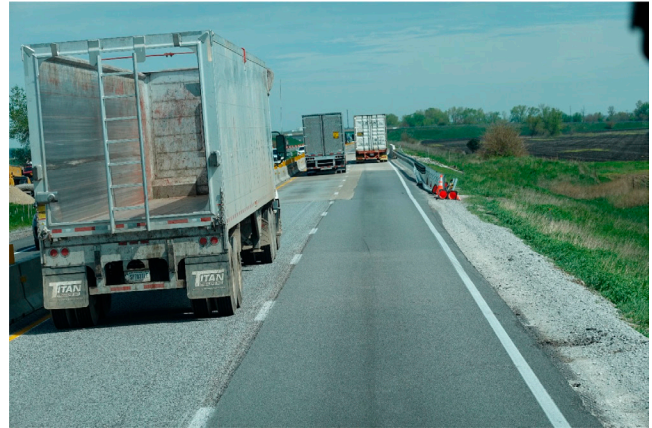
Figure 2.4 A Damaged Guardrail.
