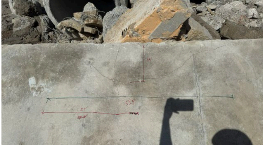
Figure 4.12: Breakout cracks in Specimen 3
