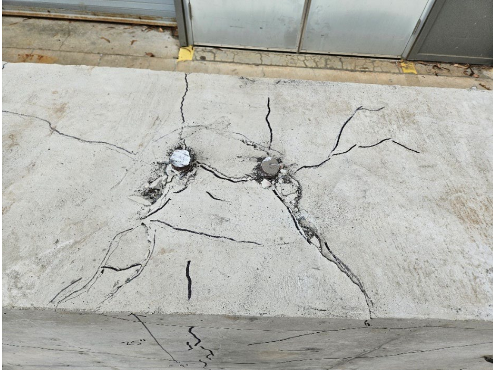
Figure 4.43: Damage on top of the concrete beam of Specimen 8
