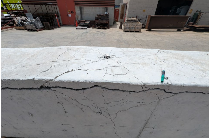
Figure 4.60: Damage on the top face of the concrete beam of Specimen 10
