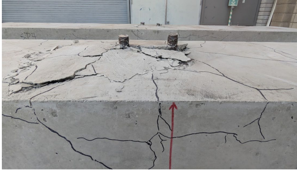
Figure 4.51: Damage on the top face of the concrete beam of Specimen 9
