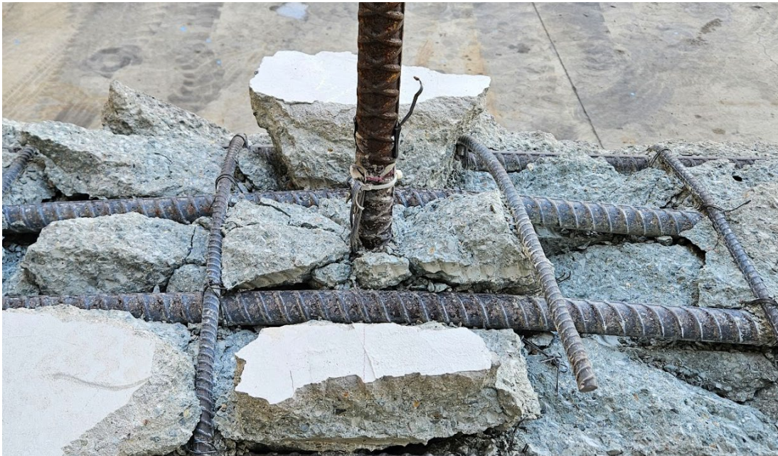
(b) Crushing in the vicinity of the headed bar
