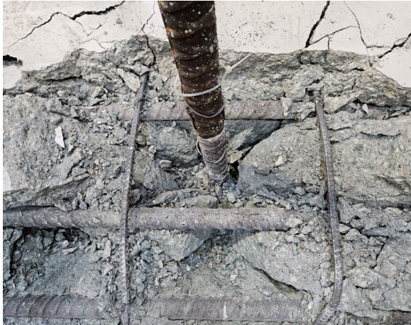
(a) Crushing in the vicinity of the headed bar
