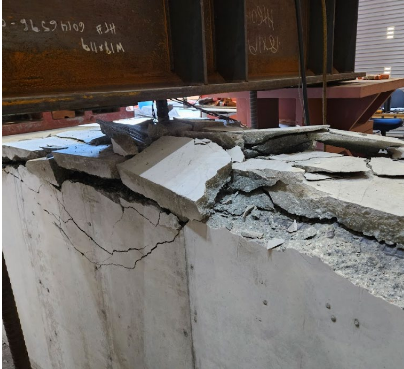
(a) Lifting of cracked concrete pieces at the surface of the beam
