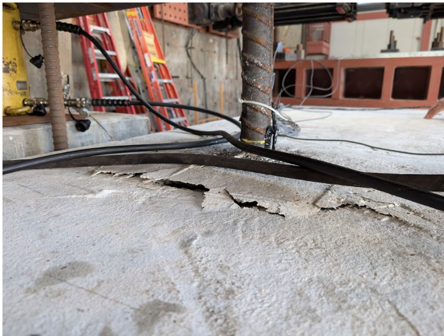
Figure 4.72: Damage on the top face of the concrete beam of Specimen 12
