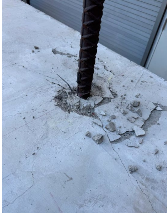
Figure 4.32: Damage at the top surface of Specimen 6
