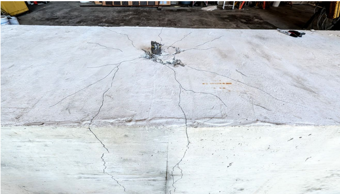
Figure 4.80: Damage on the top face of the concrete beam of Specimen 13
