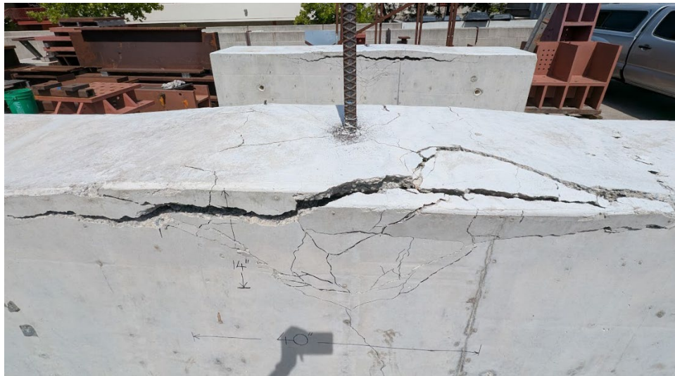
Figure 4.66: Damage on the top face of the concrete beam of Specimen 11
