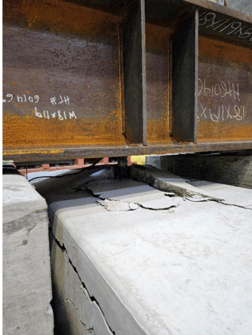
(a) Cracking at the top of the beam
