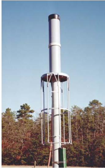
Figure 5: HK-012 Coaxial Dipole Mounted on Fiberglass Mast
