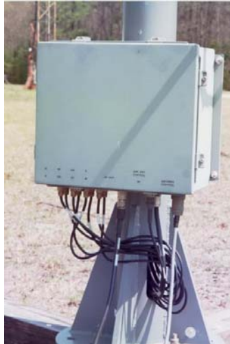
Figure 10: Control Box at Base of AA2030 Array
