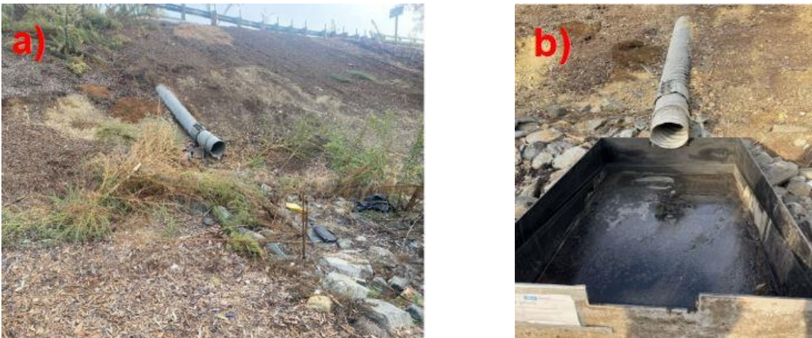
Figure 14.5 Water collection tank installation at pilot site: (a) pre-installation conditions and (b) post installation water collection tank.
