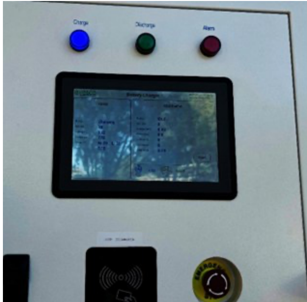
Figure B.5: Charging status display on the EVES-6060 interface during operation
