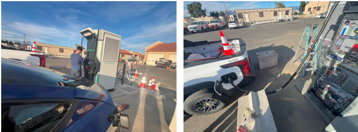
Figure 3.16: Photos showing testing FreeWire Boost Charger 200 during final commissioning process at Magaña Ortega Maintenance Yard
