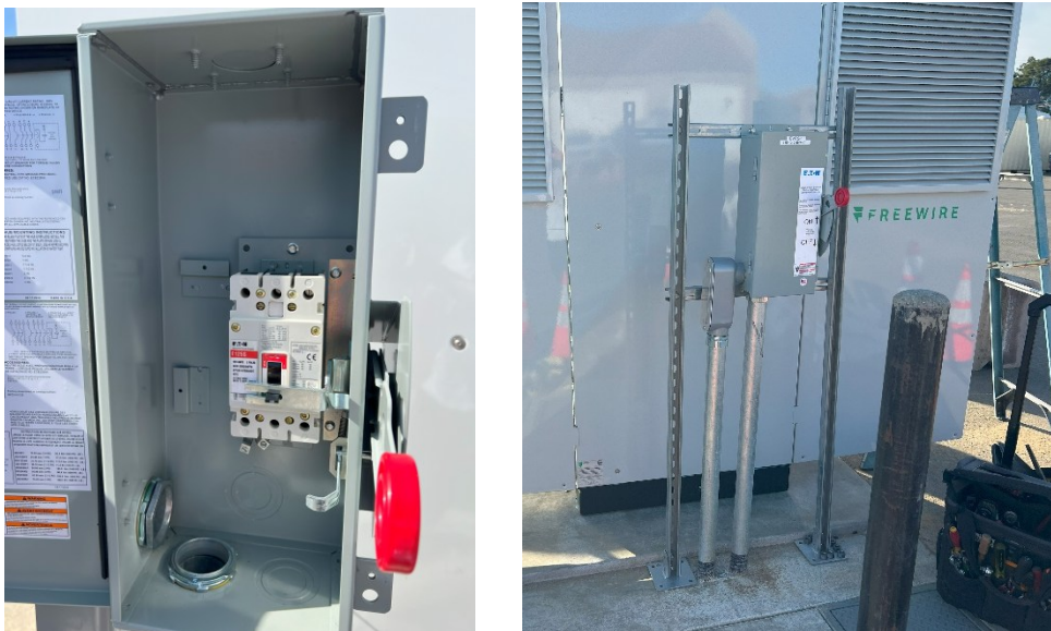
Figure 3.14: Photos showing panel installed behind FreeWire Boost Charger 200 and protective rails
