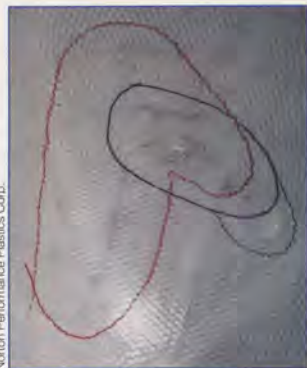
A look at the interior surfaces of a radome shows how damage inside can be greater than what appears outside. This is why thorough diagnostic procedures call for both interior and exterior examination.
