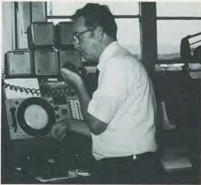
Direction finding equipment is used in most flight service station assists. Here a veteran specialist at the Martinsburg, W. Va., FSS watches the scope after punching in the frequency used by a lost pilot. Giving your frequency when you call may save valuable time, as the specialist may be handling several calls from aircraft in trouble at the same time.
