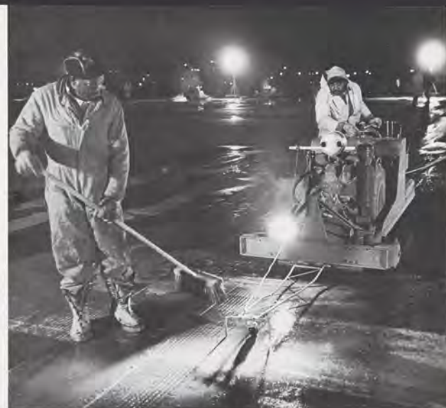
At Washington National Airport workers grooved 200 feet of runway a night in "graveyard" shift.
