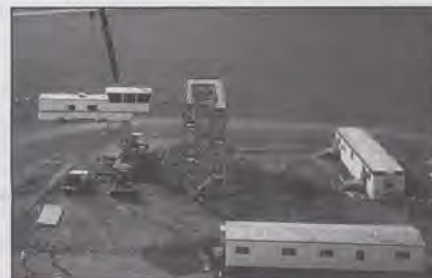
A crane lifts the mobile tower to its new home atop a 40-foot scaffold.
