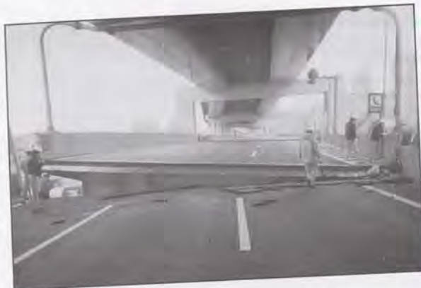
Elevated expressways, such as this one, were devastated by the Hanshin Awaji earthquake centered near Kobe, Japan, that registered 7.2 on the Richter Scale.
