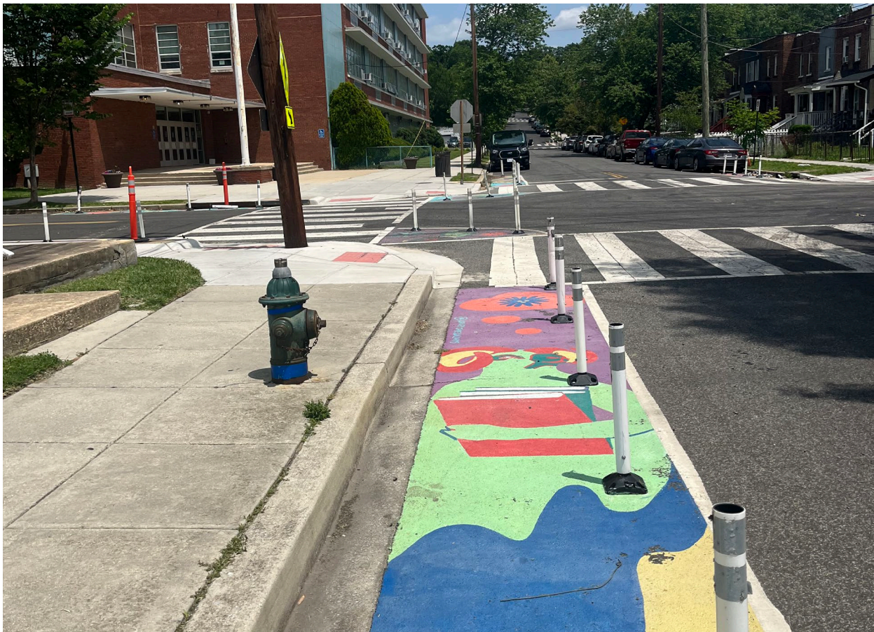
Figure 3-3 A Tactical Curb Extension with Mural Art at 56th St NE and Eads St NE
