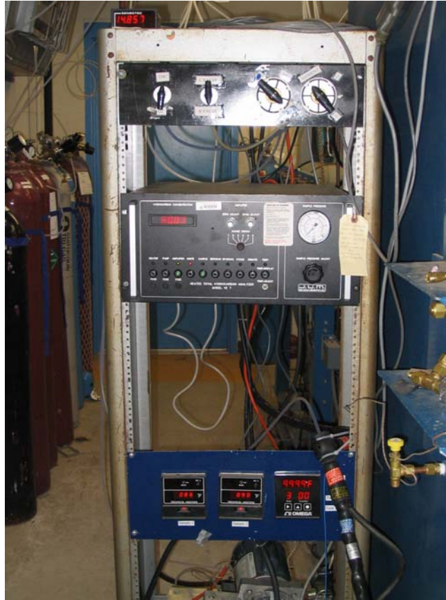
Figure 3.3. View of the instrumentation rack. From top to bottom are: Pressure transducer display, span gas manifold, hydrocarbon analyzer, temperature controller panel, and heated sample pump.
