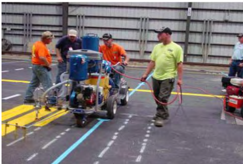
Figure 3. Application of Edge Lines on new HMA at Test Site One Inside the FAA William J. Hughes Technical Center NAPTF
