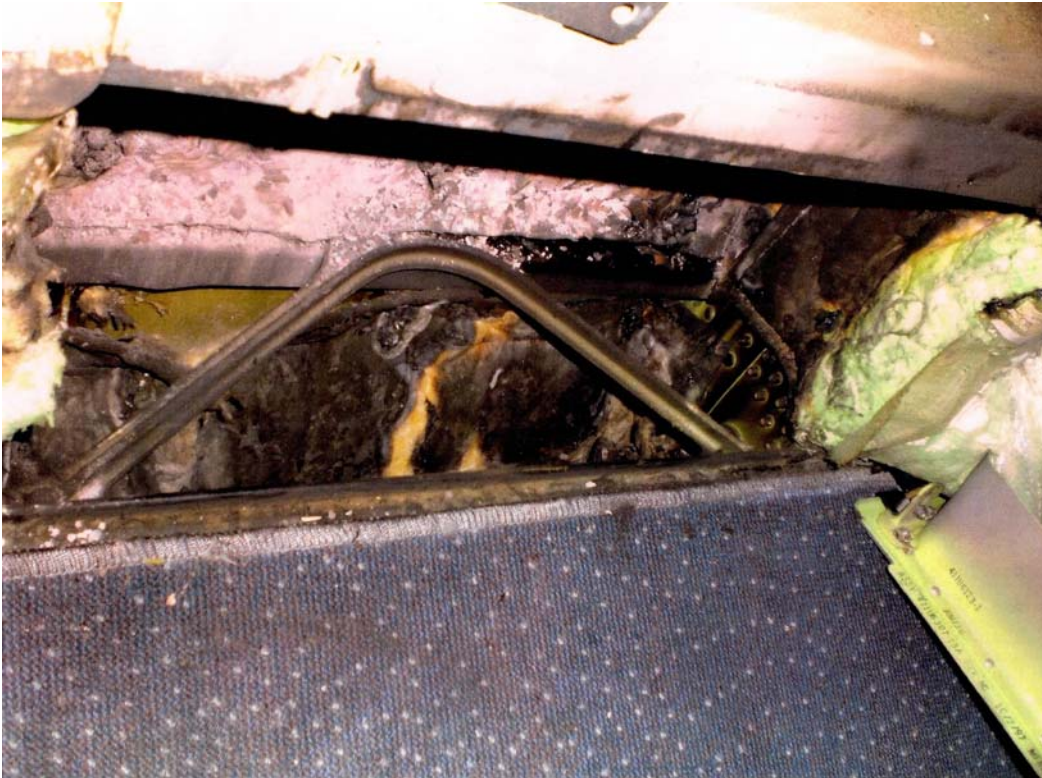
Figure 1. Burned Thermal Acoustic Insulation in the February 23, 2008, Fire Event on EVA BR67
