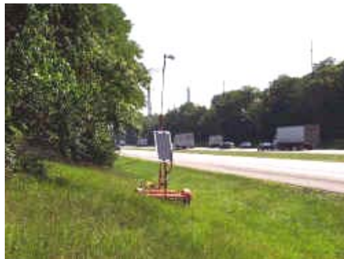
Figure 3-3 Side-Fire Microwave deployed in Springfield, IL (AIMS™/United Rentals)
