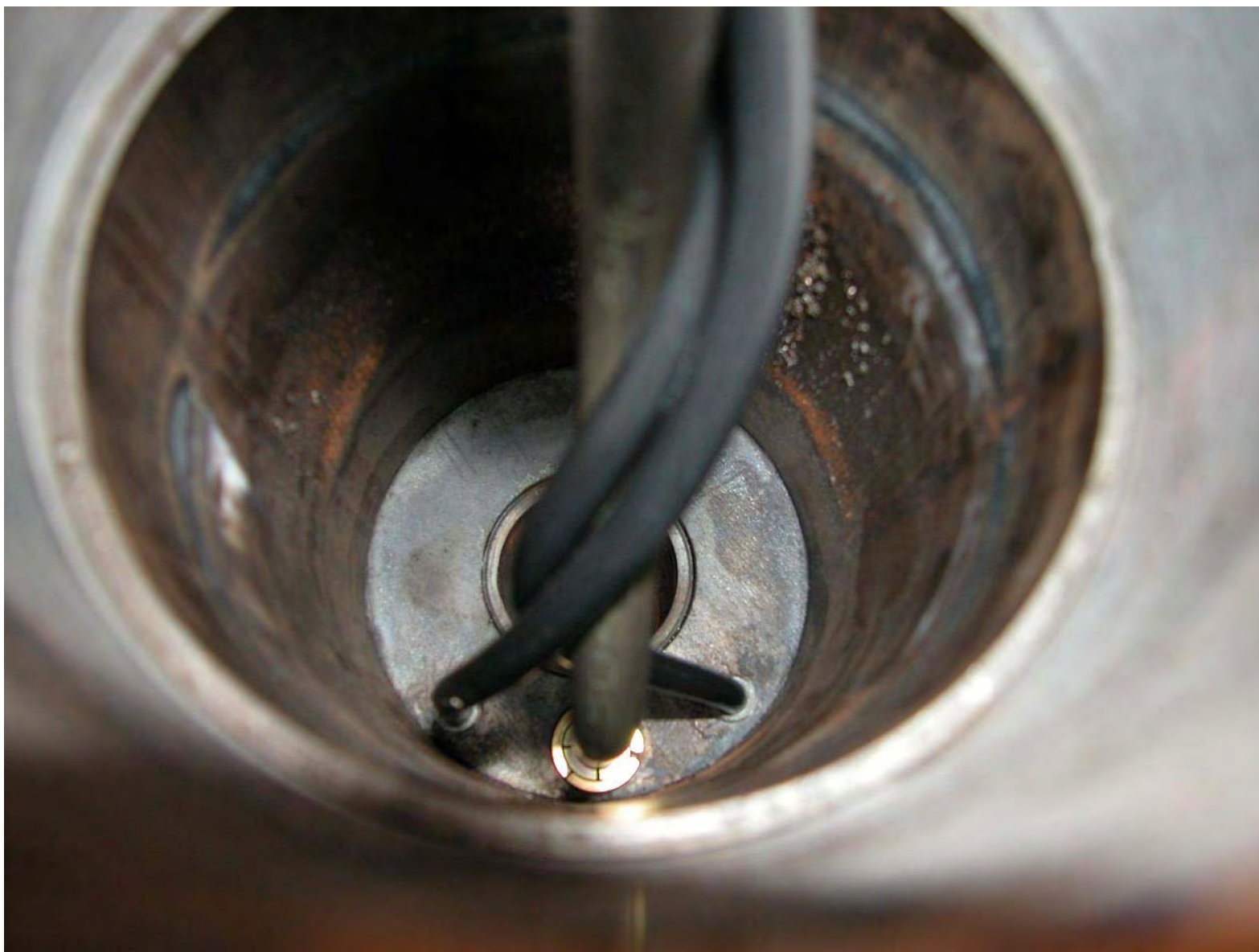
Figure A-9. Photograph of the Igniter Wires From Below
