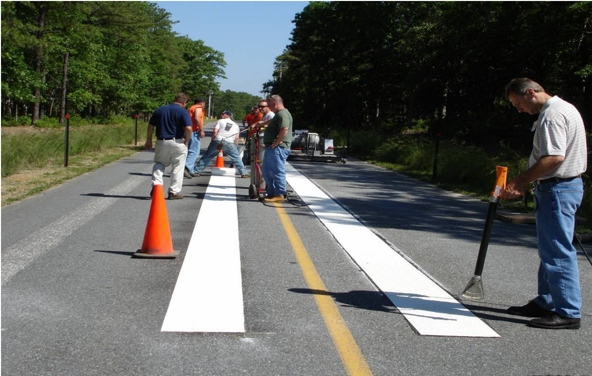
Figure 7. A 150-Foot White Stripe on HMA at FAA William J. Hughes Technical Center
