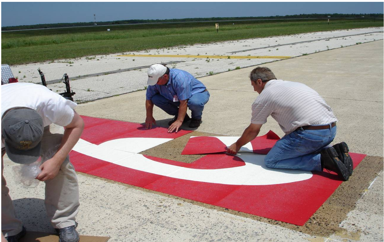
Figure 3. Aircraft Parking Location #6 on PCC at FAA William J. Hughes Technical Center
