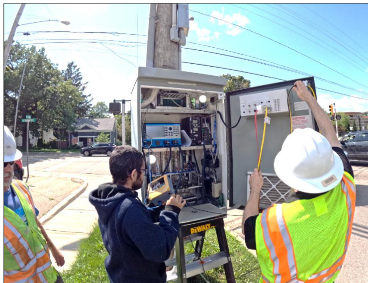
Figure 5.2 Field installation of the data diode device by the research team at an Owosso intersection in 2023 (Gowda et al., 2024)
