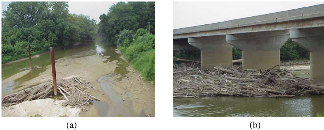
Figure 5.3: Site photographs from Aug. 17, 2000: a) view upstream of debris deflectors, b) view of piers on the left side (looking downstream) of river
