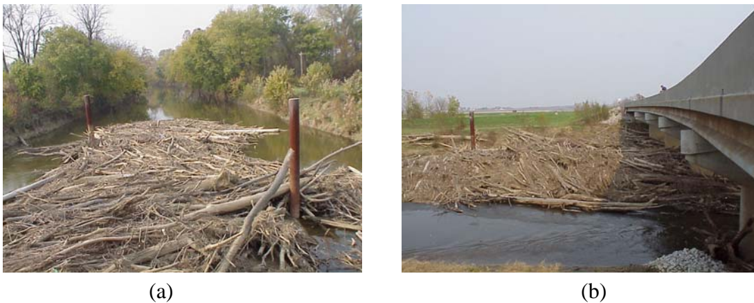
Figure 5.4: Site photographs from Oct. 26, 2000: a) view upstream of deflectors (same as Fig. 1.2a), b) view of piers on left side (looking downstream) of river
