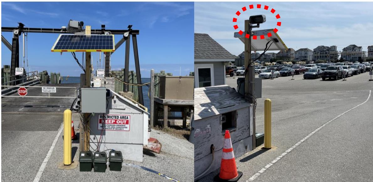
Figure 2: LPR Camera Installation on Left Dock
