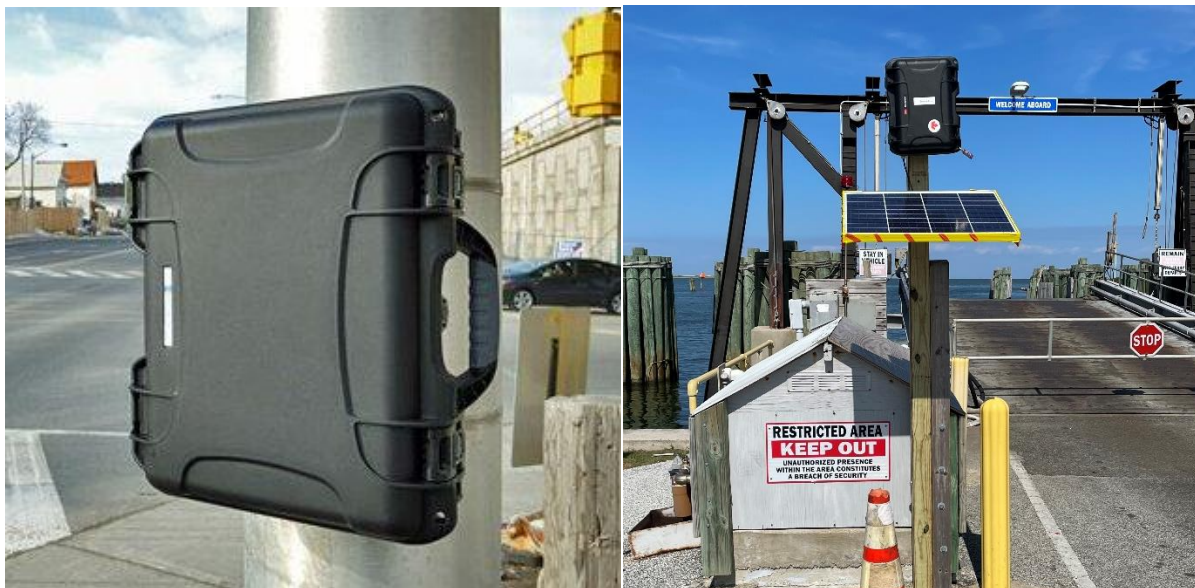
Figure 4: SMATS Hardware Installation Example (without solar panel)[left], SMATS Ferry Sensor 2 Installation [right]
