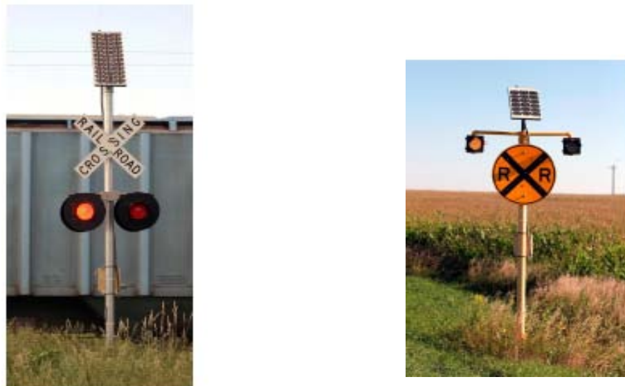
Figure 5. Mn/DOT Grade Crossing Warning Lights (left) and Advance Warning Sign Lights (right) (URS and TranSmart, 2005)
