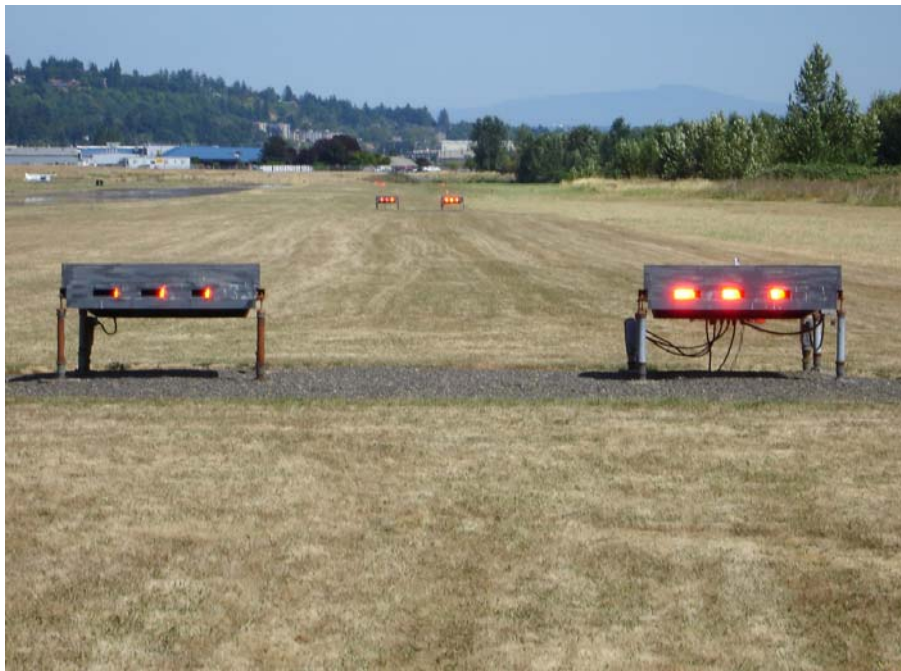
Figure B-2. The VASI Units Before Modification
