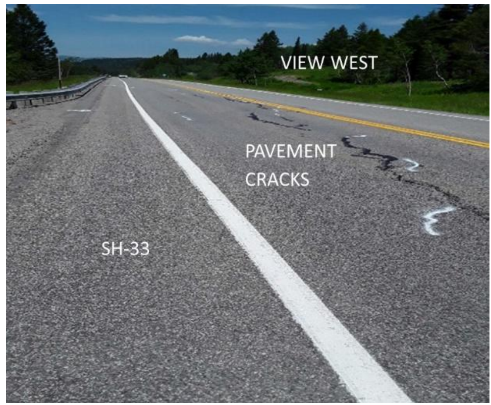
Figure 3.62 Longitudinal Cracks in SH-33 Pavement by the State Line Turnout Caused by Slope Movement between the Road and Trail Creek (photo: Shawn Enright, June 2024)
