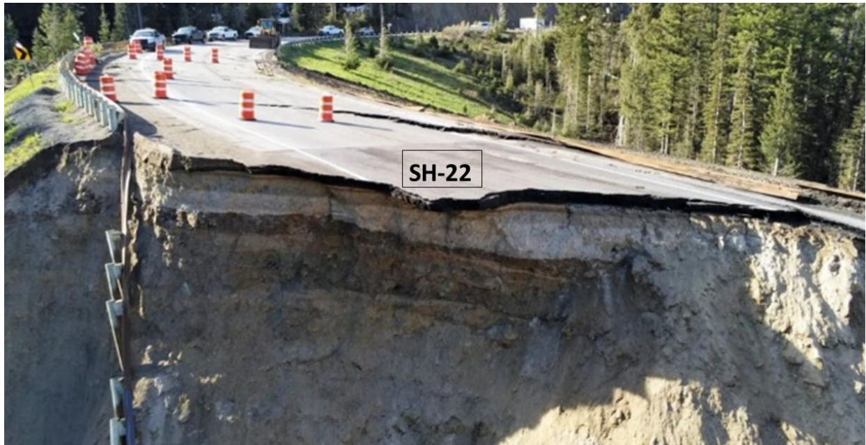
Figure 3.55 June 6 to 8, 2024 Teton Pass Landslide along the SH-22 in Wyoming (photo taken from Petley 2024).
